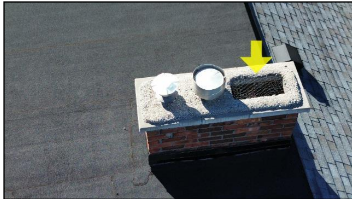
24. Rain cap missing or damaged
