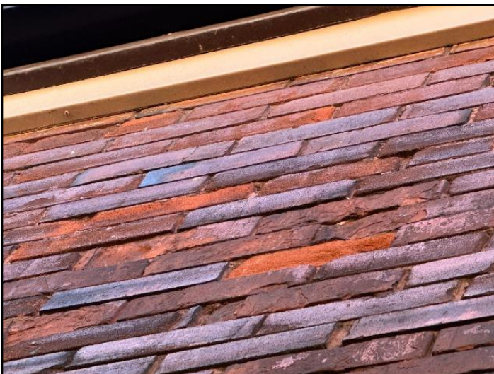
5. Minor spalling example
