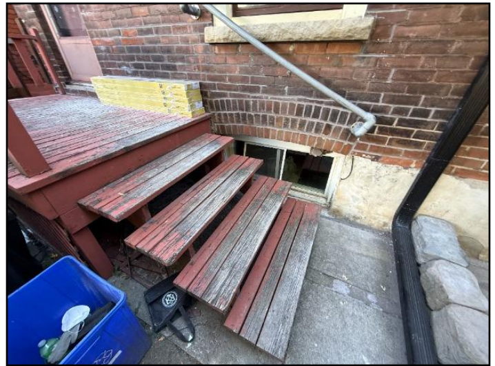
12. Wood step board not secured
