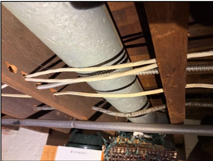
20. Too close to/touching duct, pipe, vent or...
