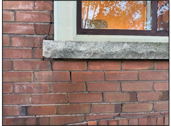
8. Typical minor cracks at front
