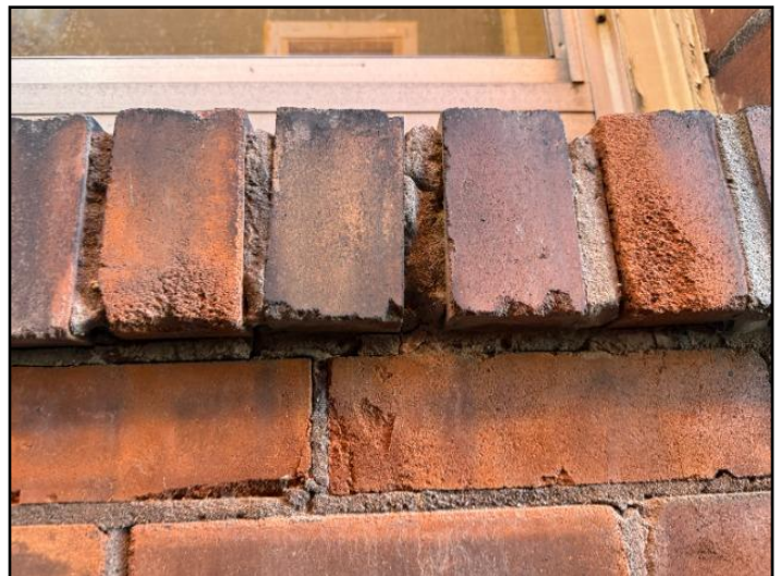
6. Typical mortar deterioration at brick sill
