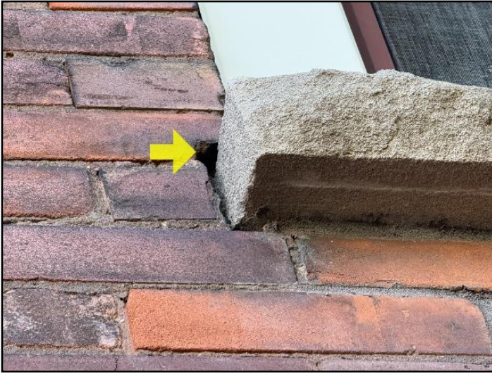
7. Missing mortar example
