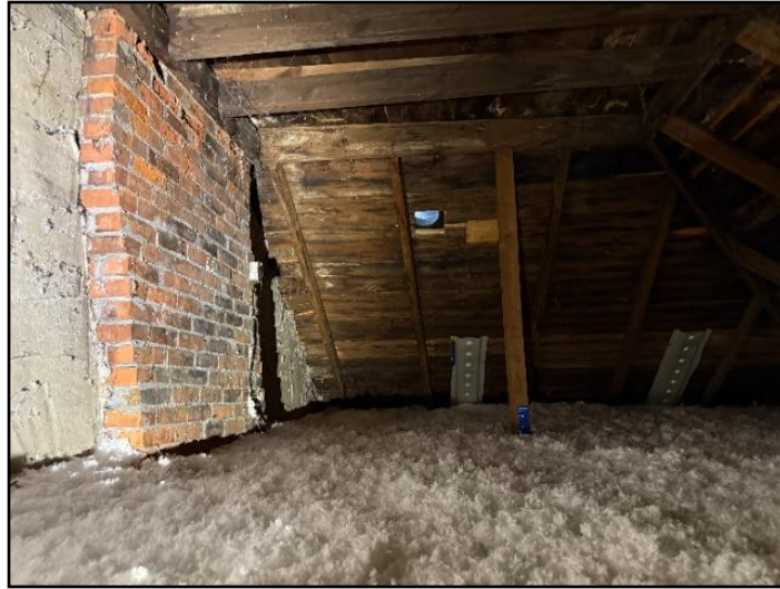
17. Water stains or discoloration - Attic plank...
