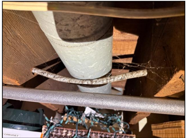
21. Too close to/touching duct, pipe, vent or...
