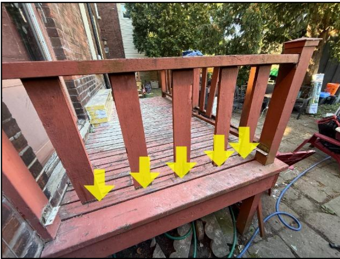
11. Spindles loose or damaged
