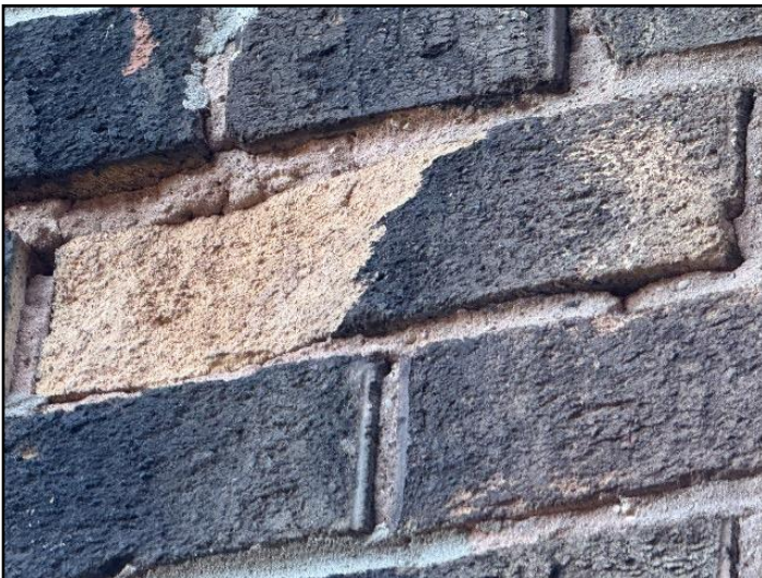
17. Masonry and/or mortar deterioration
