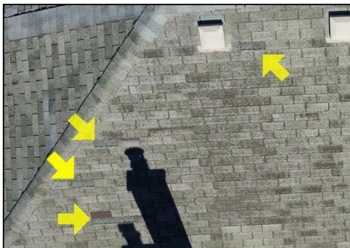
3. Missing, loose or torn
