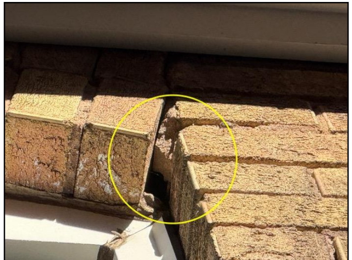
18. Masonry and/or mortar deterioration
