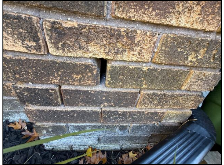
16. Masonry and/or mortar deterioration
