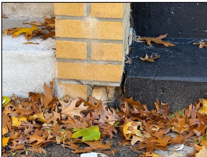
13. Masonry and/or mortar deterioration
