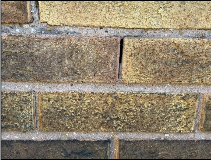
15. Masonry and/or mortar deterioration
