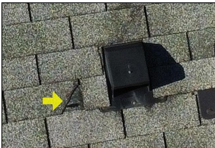
2. Missing, loose or torn
